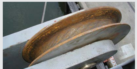
Contact with rusted, uneven surfaces will shorten the service life of synthetic lines due to abrasion and cutting damage.
