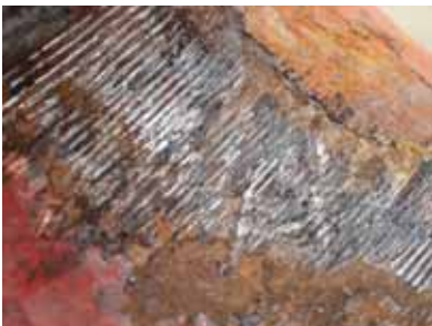
TOP: Typical condition of the load barrel winches when working with wire rope.
